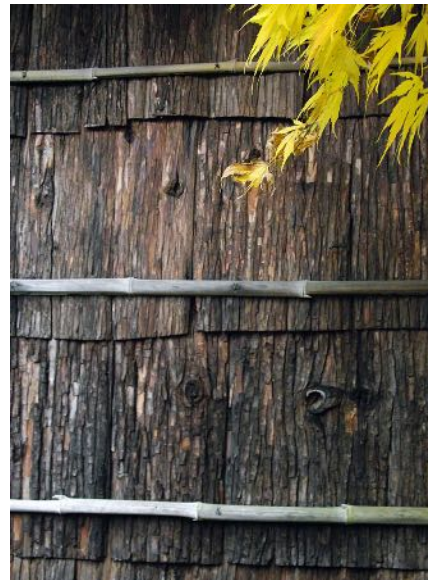
Figure 5 Bark and bamboo cover the storage boxes for the outer shutters when not in use.
